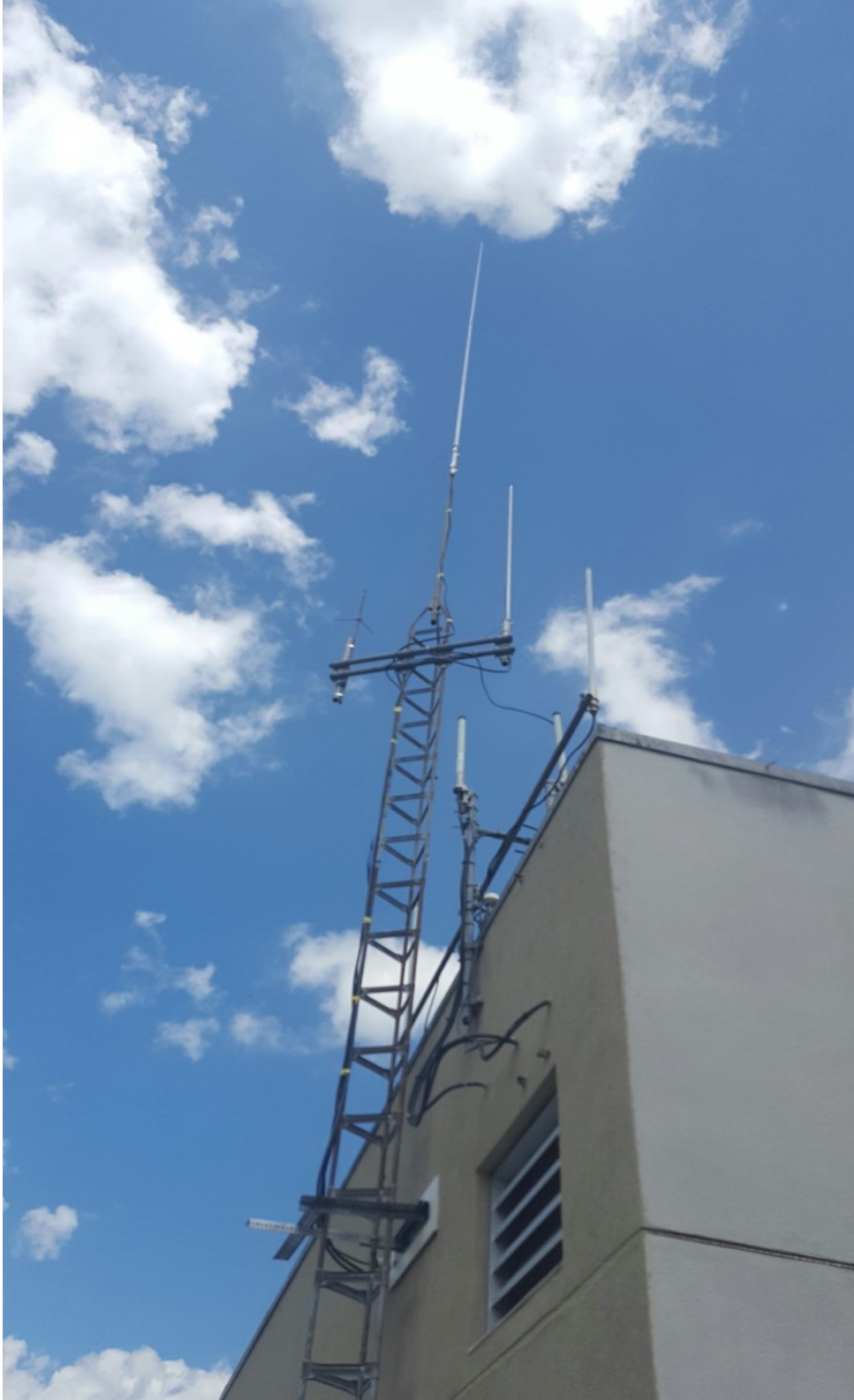
MARA's Tower and Antennas as Installed on the Hospital "Penthouse". ABIGF photo
