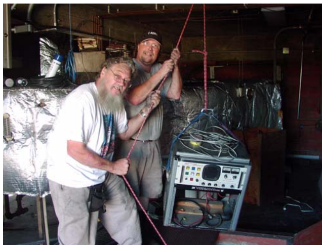
above: K1YTS and AB1GF prepare to lower the cabinet through the floor to the floor below.
