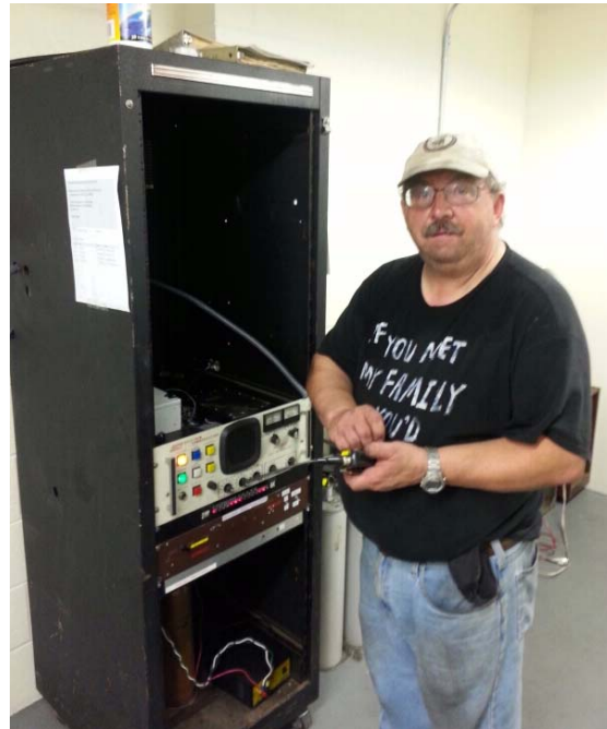
above: KD1YH with the repeater installed in its new rack.
