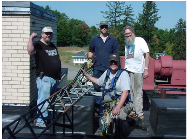
above: KD1YH, KB1YRS, K1YTS and AB1GF have the tower down ready to carry across the roofs.
