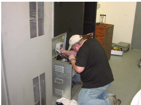
below: KD1YH removed the repeater from the old cabinet.
