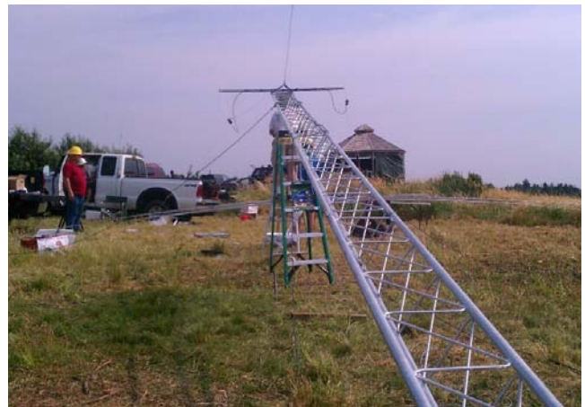
Above: the top of the tower is supported on a ladder while the rotator is installed.
